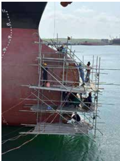
Figure 3 M.V. Courtesy K, undergoing bow damage repairs while afloat at Hambantota
